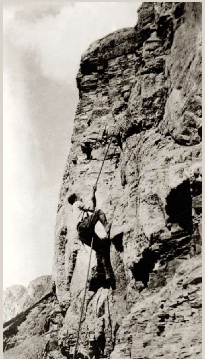
FIGURE 17.18: Road workers defied their fear of heights to build the Granite Peak retaining wall. Some people call the Going-to-the-Sun Road the “crown of the continent.”
