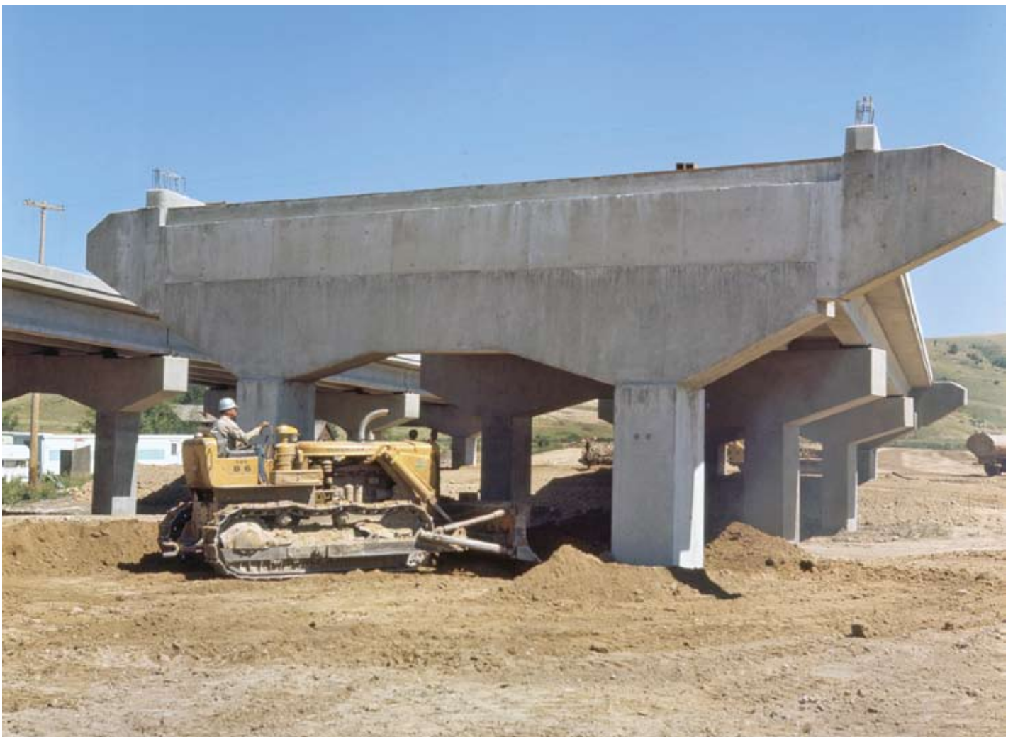
FIGURE 20.17: A worker bulldozes ground during construction of Interstate 90 near Bozeman. Montana had never had roads like this before. Interstates changed the landscape, brought in tourists, and also allowed long-distance travelers to zip right through Montana, stopping just long enough to fill up with gas.
