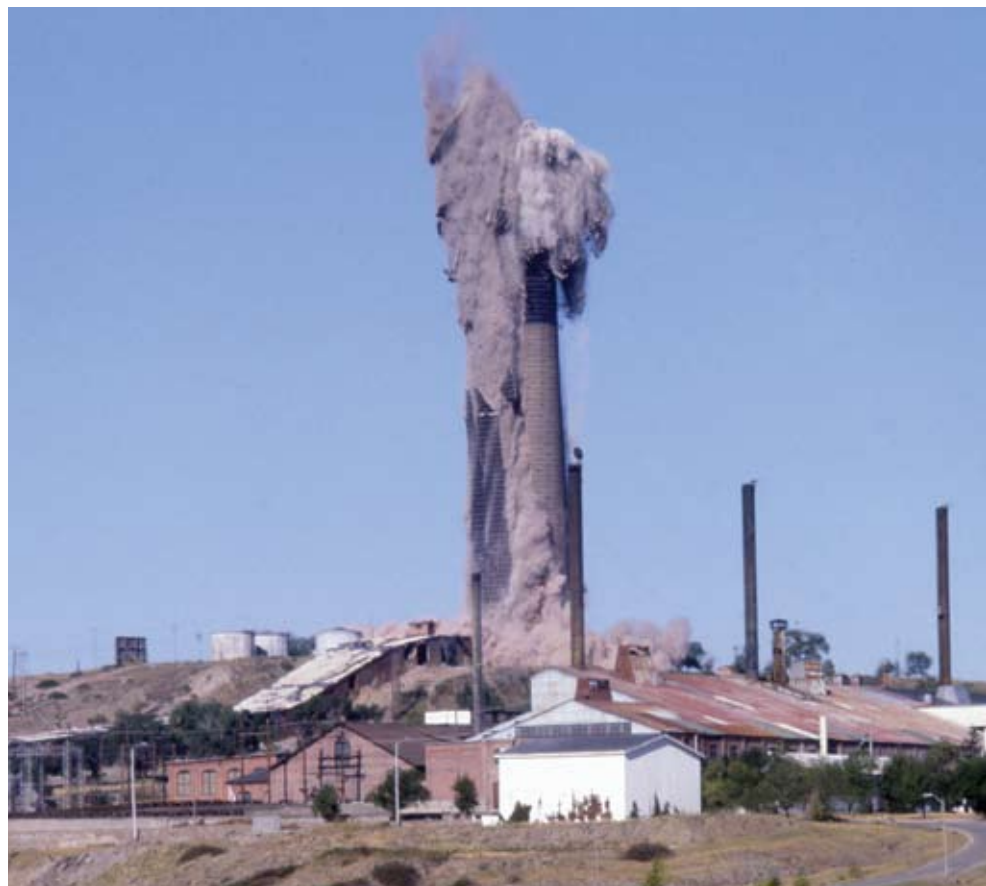
FIGURE 22.5: ARCO shut down the Black Eagle refinery in 1980. On September 18, 1982, an explosives expert demolished the 506-foot-high brick smokestack. A crowd of 40,000 watched it go and said good-bye to 70 years of smelting jobs in Great Falls. "When the stack came down it was heartbreaking," said George Rimmel, who worked there 42 years. "It was a landmark, just as much as the Statue of Liberty."
